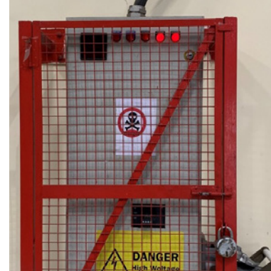
Working with High Voltage
